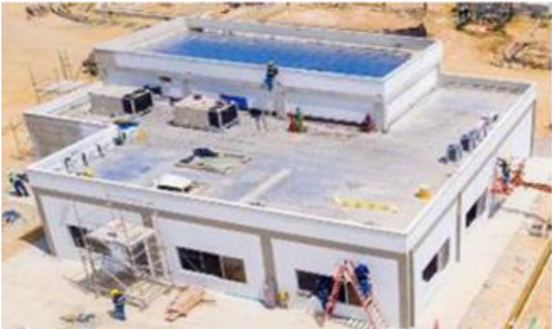
Administrative Building and Control Center - August 2016
