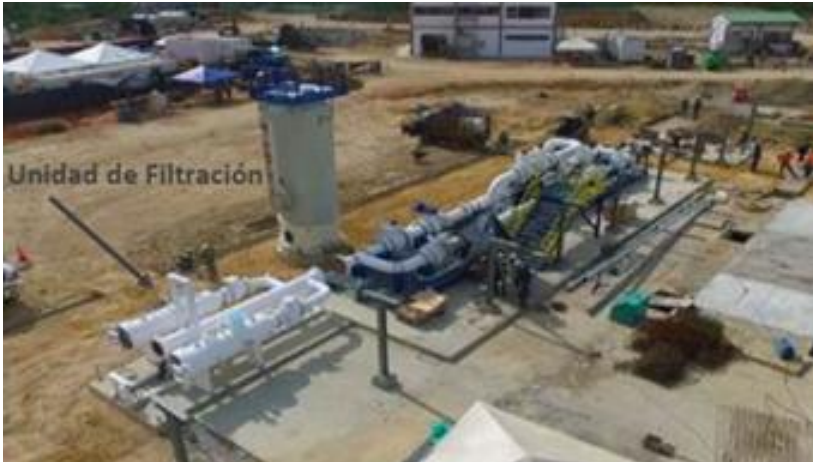
Installation of measurement and filtering units - August 2016
